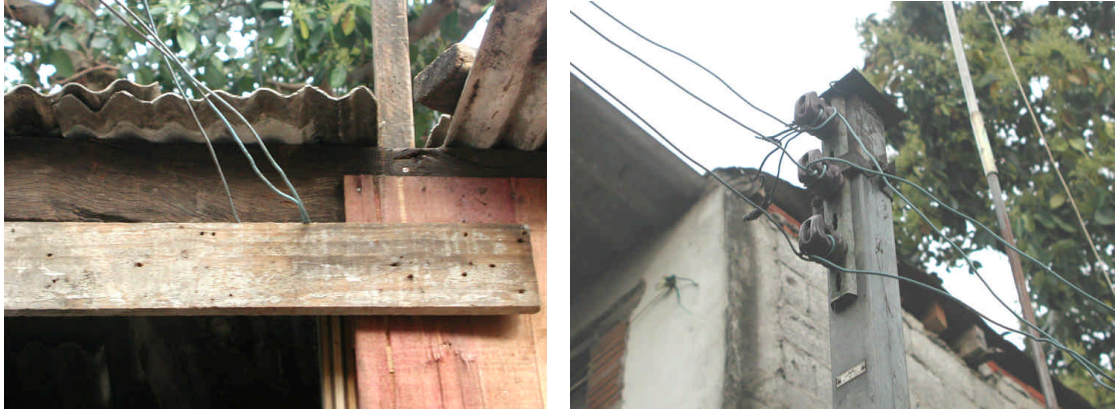
Figure 2. Unsafe energy connection pictured by the students
